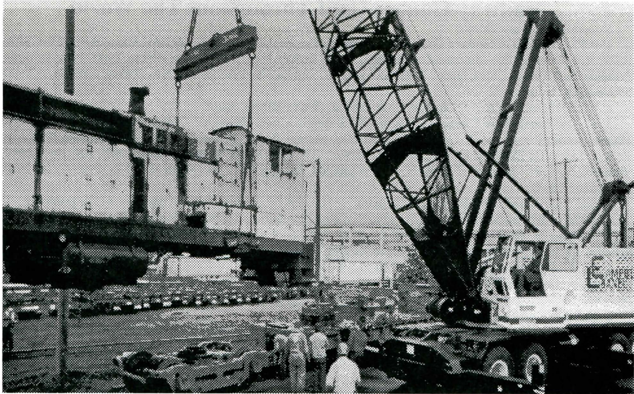
Peter Rodabaugh gives instructions to David Stimac to position the second truck under the Alco. After the truck was in position, Richard Gray and Roger White remove the chain tying it to the DODX flat car. After everyone has cleared of the locomotive, the 150 Ton crane will lower the locomotive down onto its truck.
