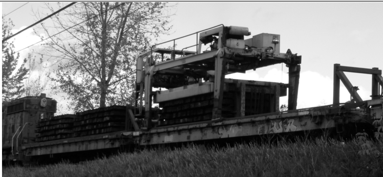
November 9 th just north of Durham Road showing the on-board tie transporter gantry which rides on rails between multiple flat cars. In this picture the gantry is unloading old wood ties, it will now move forward and pick up a load of concrete ties for delivery to the P811 which is to the right of this picture. Photo by Arlen Shel Drake.
