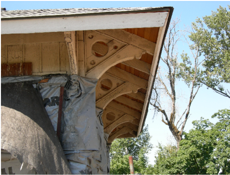
1889 Freight Depot/Baggage Shed showing triangular, scroll-sawn brackets, July 24, 2006. (Photo by Arlen Sheldrake)
