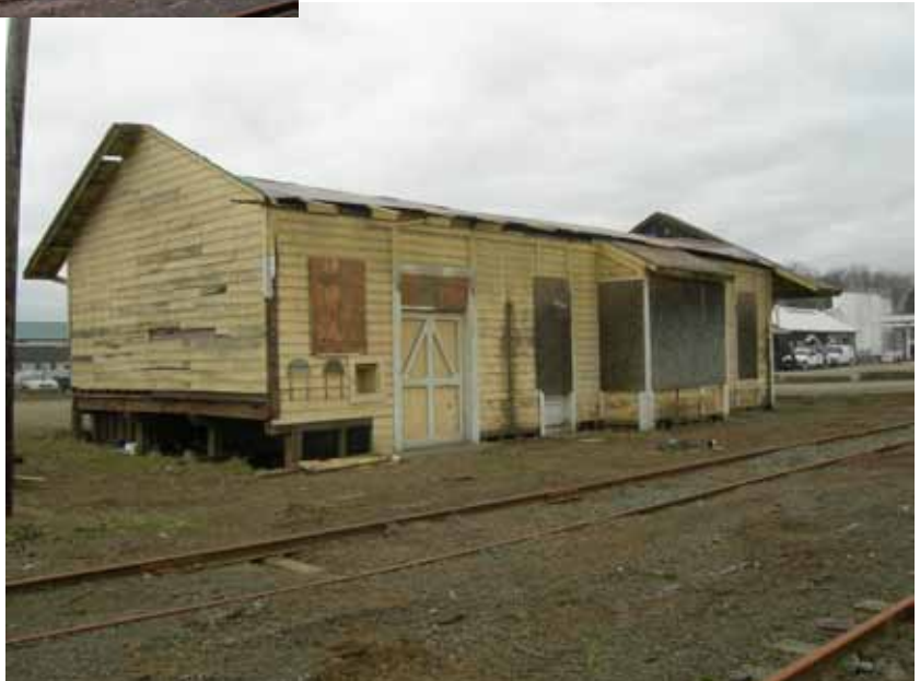
Roof and windows removed, the depot stood at its previous location, awaiting lifting and transportation.
