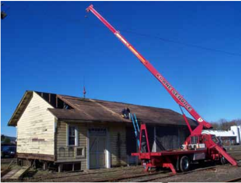
In preparation for the move, the roof of the depot had to be removed. A crane allowed the clean removal of all of the roof joists and covering.
