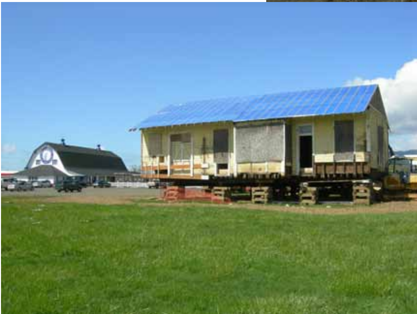
At its new, permanent location at the Blue Heron French Cheese Company facility, the depot still needs a new foundation and replacement roofing.
