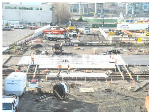
OPR Track and Water Ave. run left-to-right Future TriMet Max Tracks top-to-bottom
