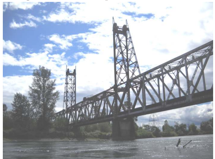
The Oregon Electric (Now Portland & Western) Lift Bridge over the Willamette River in June 2013 (Photo by David Dowrie)
