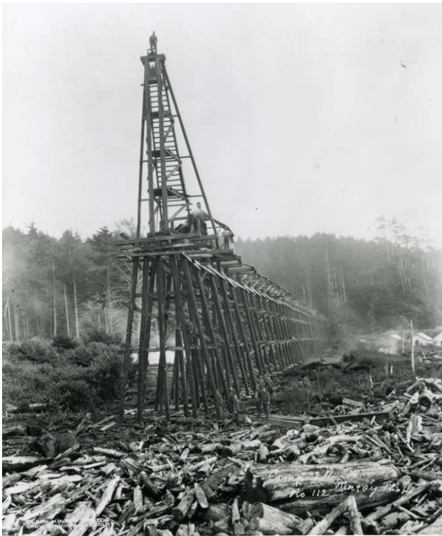
Surrounded by beach logs, one of the large trestles is being built along the coastline north of Agate Beach. Clark Kinsey No. 112
