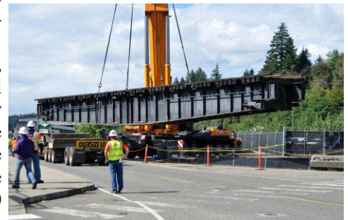
the turntable is being lifted out of the pit and swung onto a heavy haul truck.
