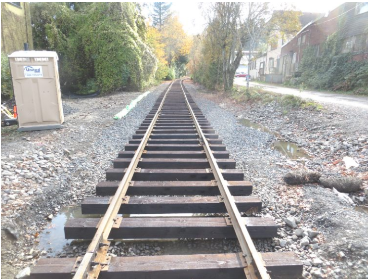
As Multnomah County's major Sellwood Bridge replacement project winds down, so does the need for using the Willamette Shore Trolley line as a project haul road. This November 3, 2016 picture shows the newly reinstalled rail line before ballasting.....expect the Willamette Shore Trolley to be again running to the South Waterfront station in 2017. (Photo by Arlen Sheldrake)
