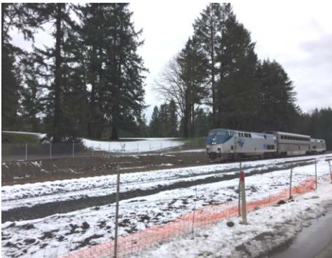
Construction of the new tracks and signals running from South Tacoma to Nisqually is nearly complete. Testing along this corridor was undertaken for mid-January through February. During this testing phase, trains will be running at varying speeds, up to 79 mph. Picture taken at the Mounds Rd and old Nesqually highway overpass.
