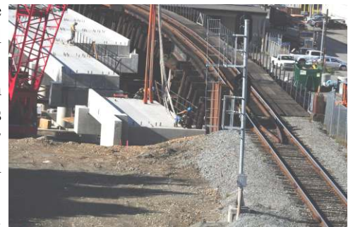
Construction of the new concrete bridge next to the MILW timber trestle (Photo by Gordon Russ)
