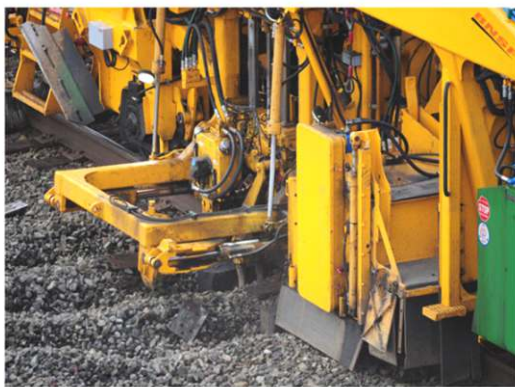
Close up of tie squaring and tamping machine. Note the tie plates on the ground.
