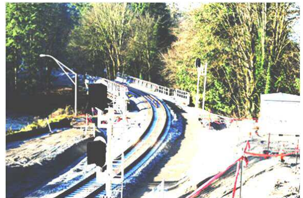
Track completed over I-5 highway and just waiting for signal and clean up completion.
