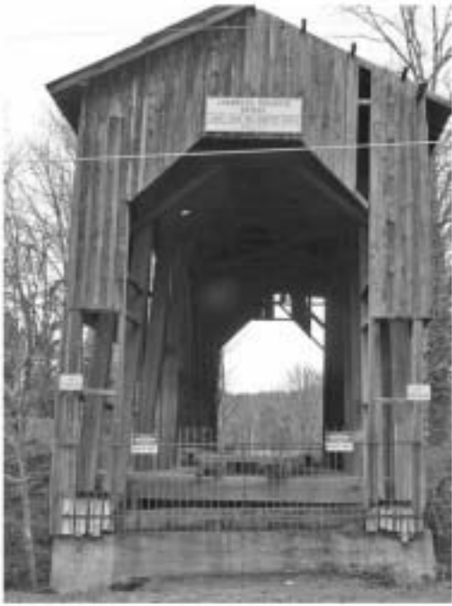
Above: The tilt of the structure is clearly shown in this photo taken in 2009, prior to disassembly of the old bridge. Rot above the piers on the upstream side caused the bridge to take on a decided list.
